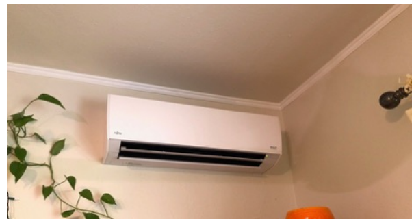
My indoor “air handlers” are ceiling mounted, but there are also floor-mounted ones.
